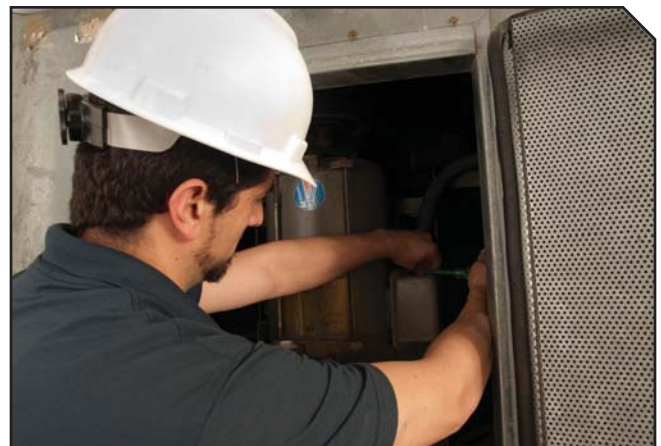
FIGURE 2. HVAC equipment with installed UV-C lamps should have an interlock switch that turns off the UV-C lamps when the door is opened. (Image courtesy of UV Resources.)
